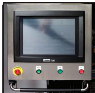
Rear Auxillary Control Panel
